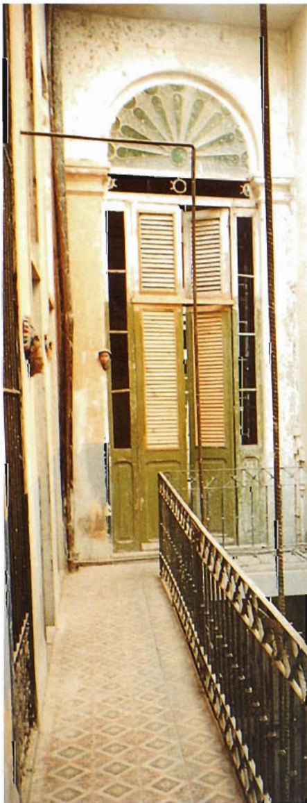
MALECÓN N° 27. INTERIOR OF BUILDING BEFORE REHABILITATIONS IN THE MALECÓN Malecon Project Cuba+Spain. Seville
